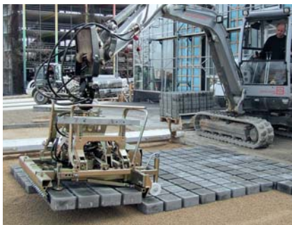
... paving even large areas with an excavator is extremely easy – Hydraulic Installation Clamp HVZ-GENIUS.
