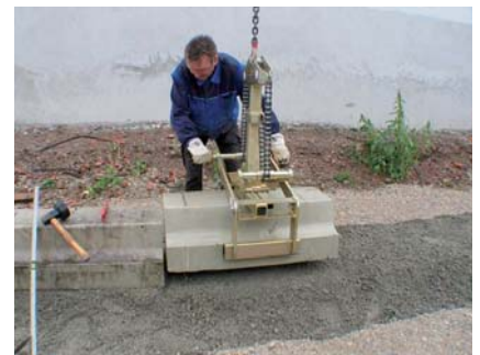
... installing heavy kerb stones and concrete elements: mechanical, powerful and safe – Grab for Prefabricated Concrete Products FTZ-UNI.
